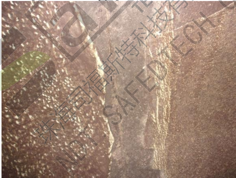
Coating Failure at a concrete joint
