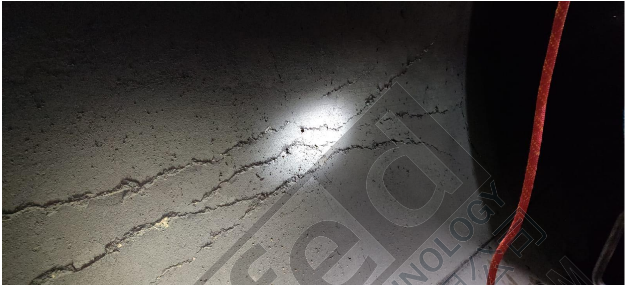
Axial Cracking on the concrete line pipe
