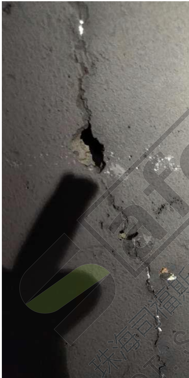
Cracking and Pitting on concrete liner
