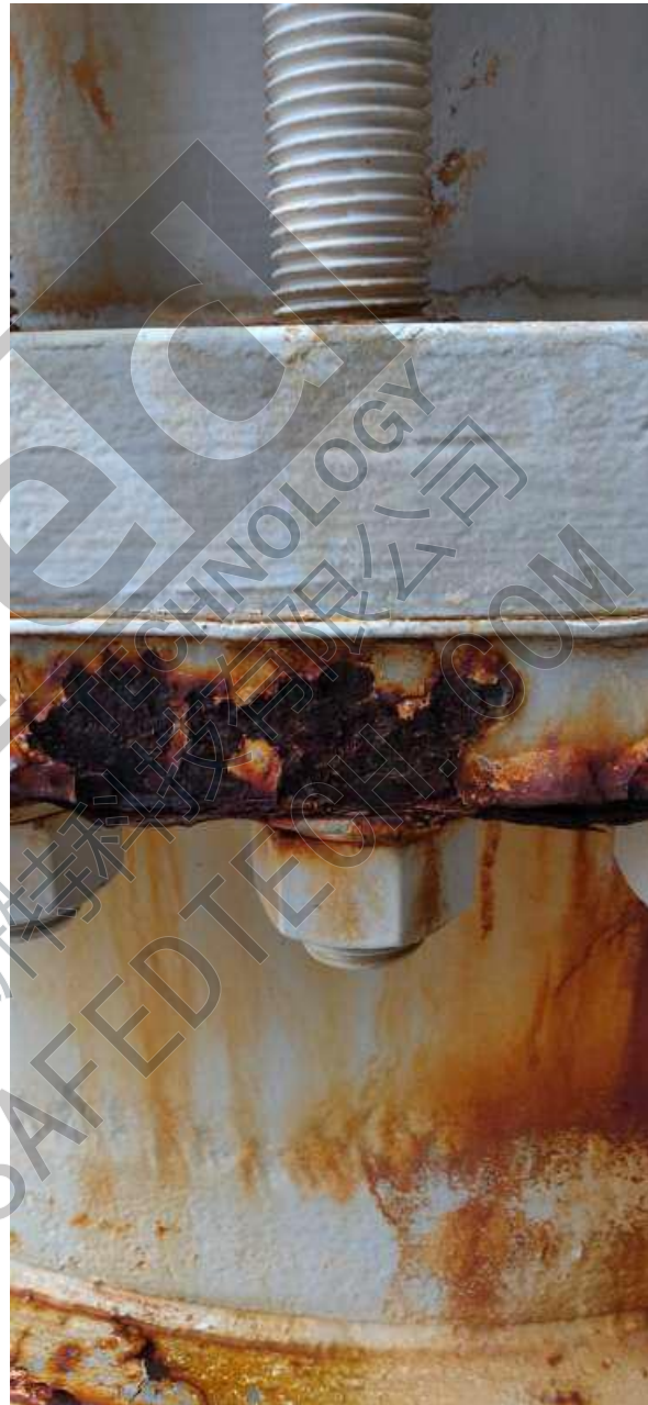
Corrosion Deterioration at flange
