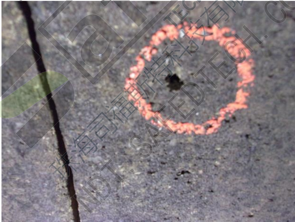
2" deep pit in concrete
