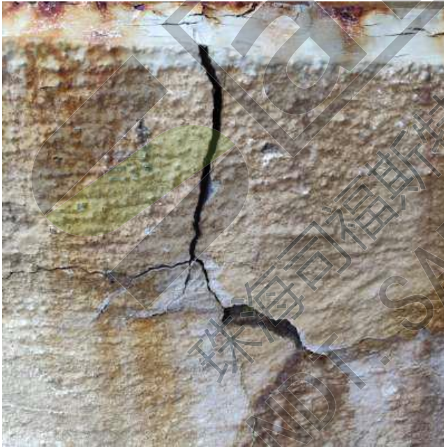
Deep Mortar Cracks on a Riser Pipe
