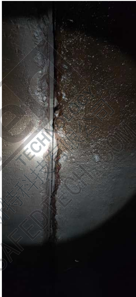
Cement Gap at a Joint
