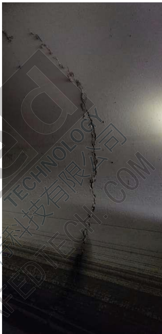
Circumferential Crack between joint 1 & 2
