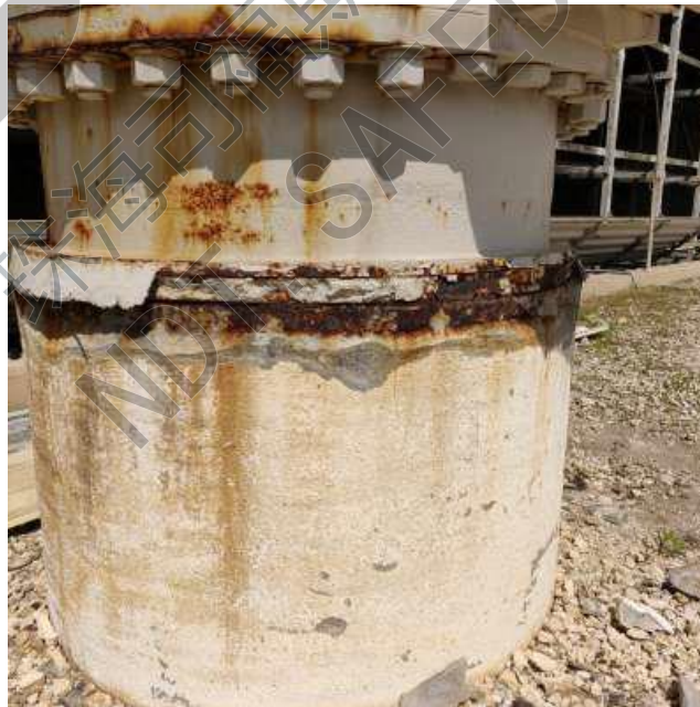
Mortar Coating failure on Riser B
