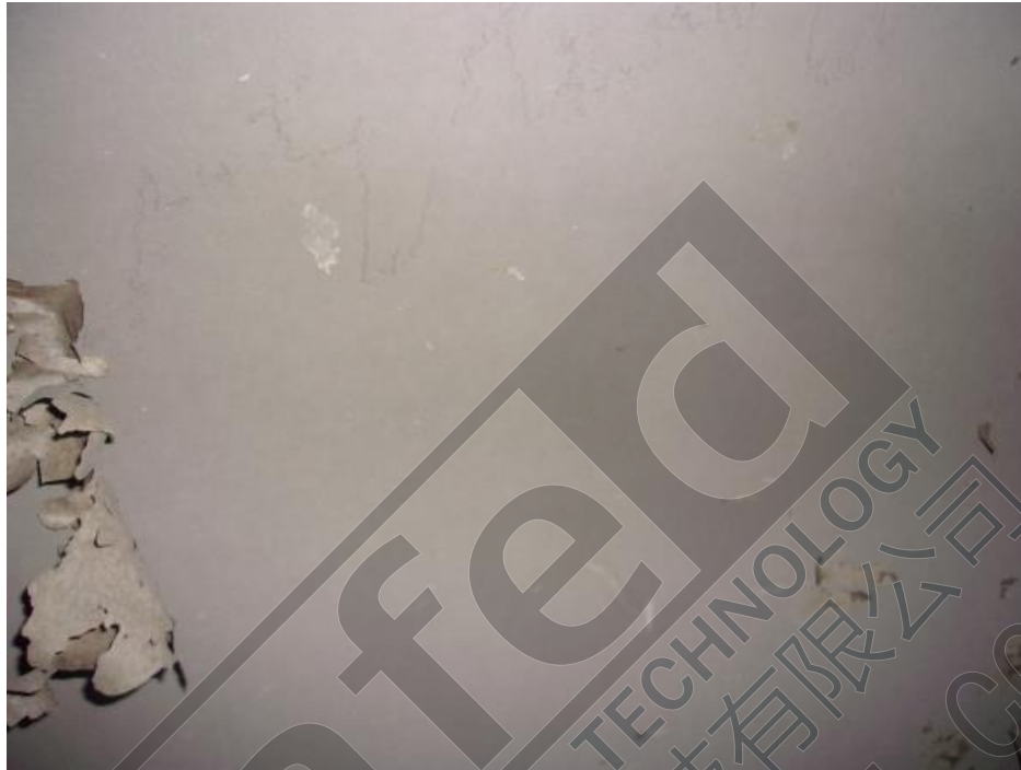
Coating on carbon steel section of pipe
