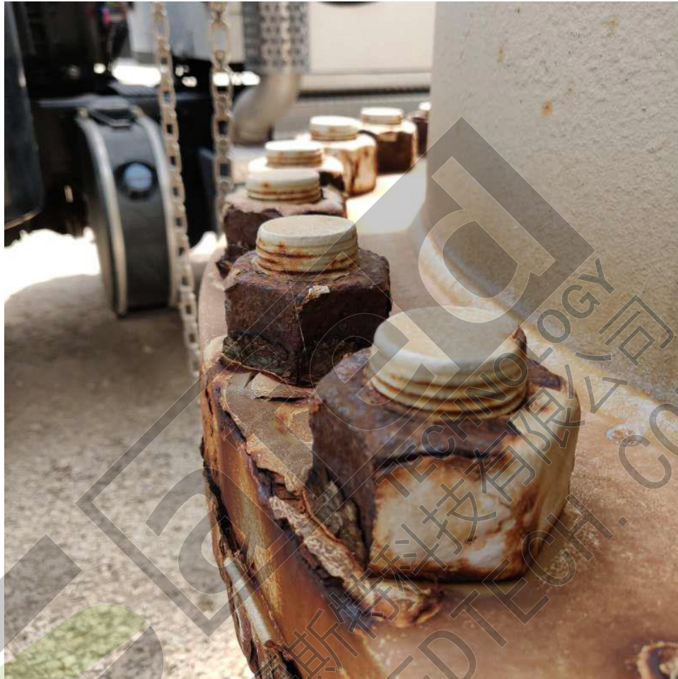
Severe bolt corrosion on flange
