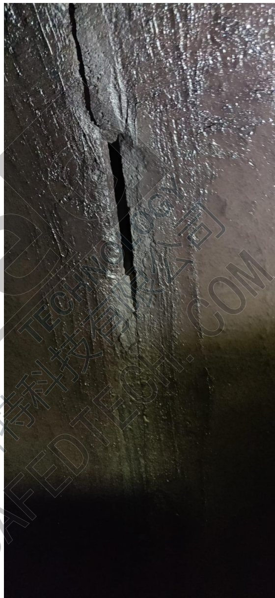
Concrete Gap at Joint
