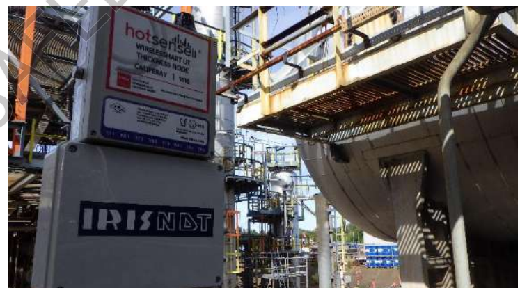
HotSense CALIPERAY Wireless UT Monitoring System
